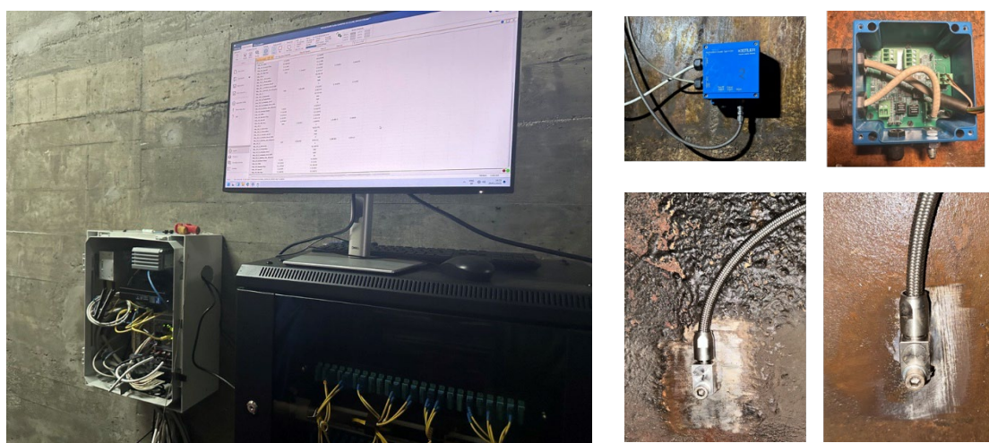
Figure 2. Monitoring cabinet and PC, sensors and coupler boxes at Valeira Power Plant.
